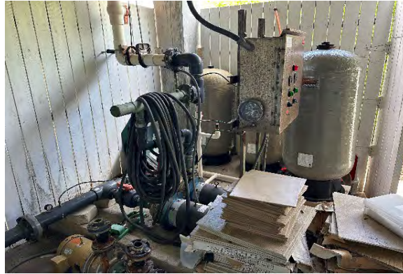
Annex Building Domestic Water Station
